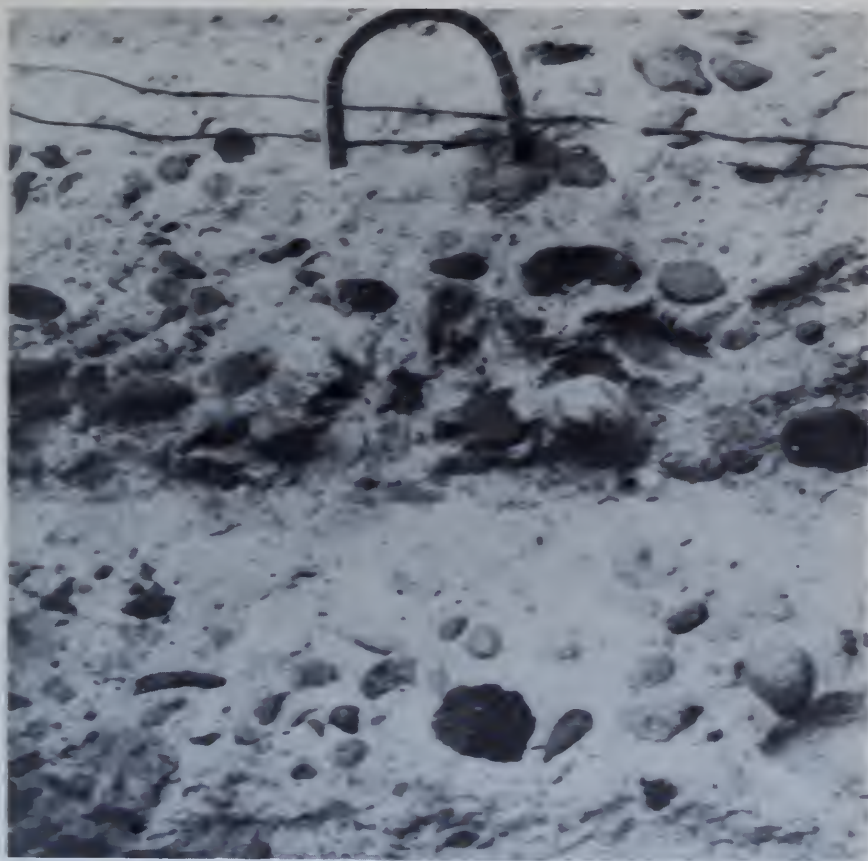
Figure 119.—Segregation in overwet concrete at fill planes, resulting in weak, porous joints subject to early weathering. PX-D-11747.
